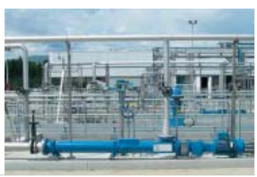
I pump for lime milk dosing
