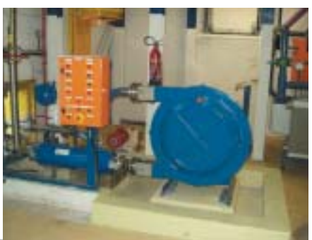
DSC pump for enamel transfer in a can coating factory
