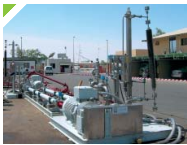
Onshore pre-commissioning of High Pressure Oil re-injection pump : 900THP100 model with API 53 plan (4'000 bfpd @ 100 bar)
