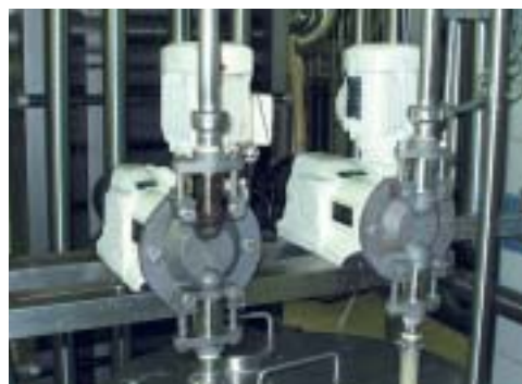
Two Préci Pump Lagoa Series pumps in the dairy industry: pumps with stainless steel body for dosing acid and soda in the Cleaning In Place zone
